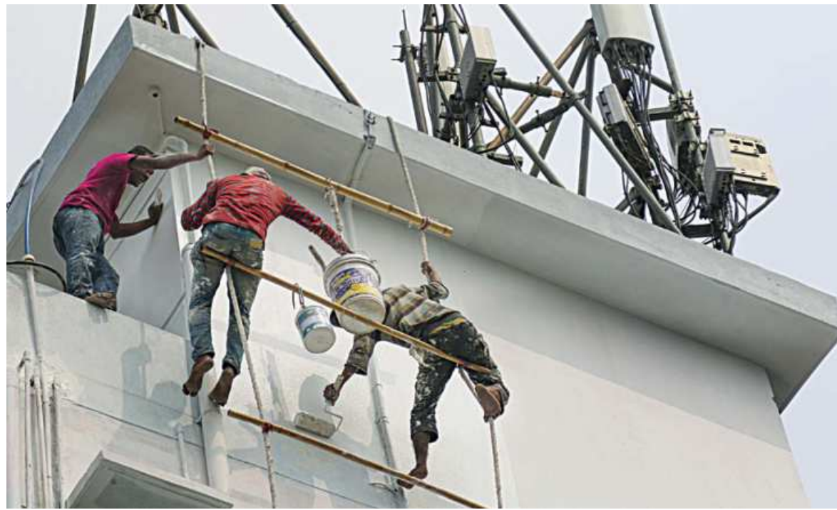
Two building painters putting their lives at risk, hanging off a makeshift ladder without any safety harness. Such disregard for safety leads to injuries and deaths. The photo was taken from For's Lake area of Zakir Hossain road in Chattogram yesterday.
