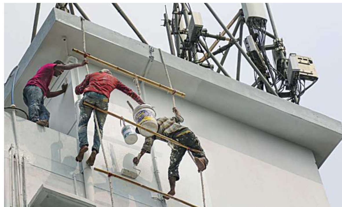
Two building painters putting their lives at risk, hanging off a makeshift ladder without any safety harness. Such disregard for safety leads to injuries and deaths. The photo was taken from Foy's Lake area of Zakir Hossain road in Chattogram yesterday.
