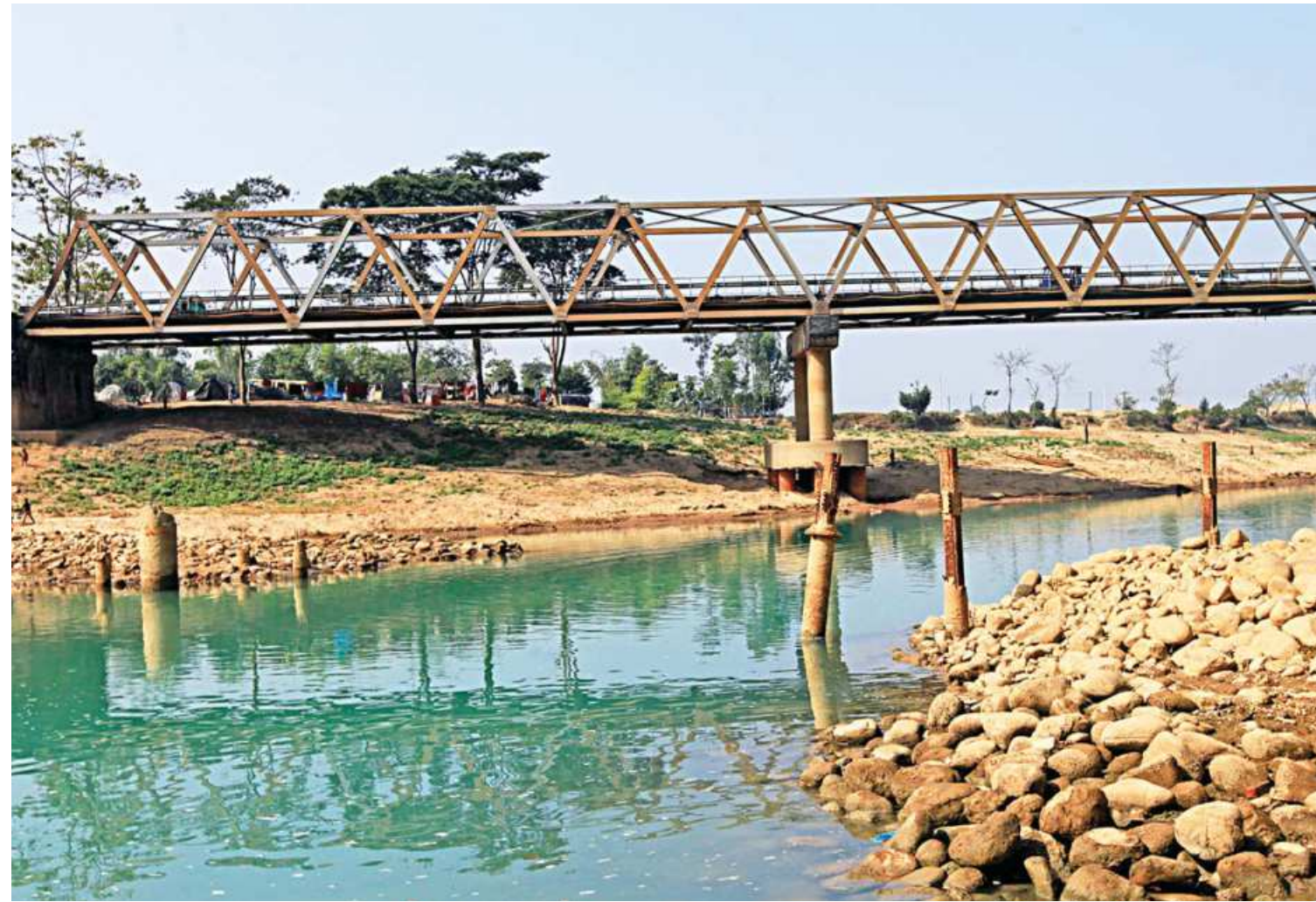
The authorities did not remove the remains of a decommissioned bridge on the Sylhet-Shillong highway even though a new bridge was built around 20 years ago. The pilings have helped reduce the navigability of the river which has shrunk significantly over the years.
