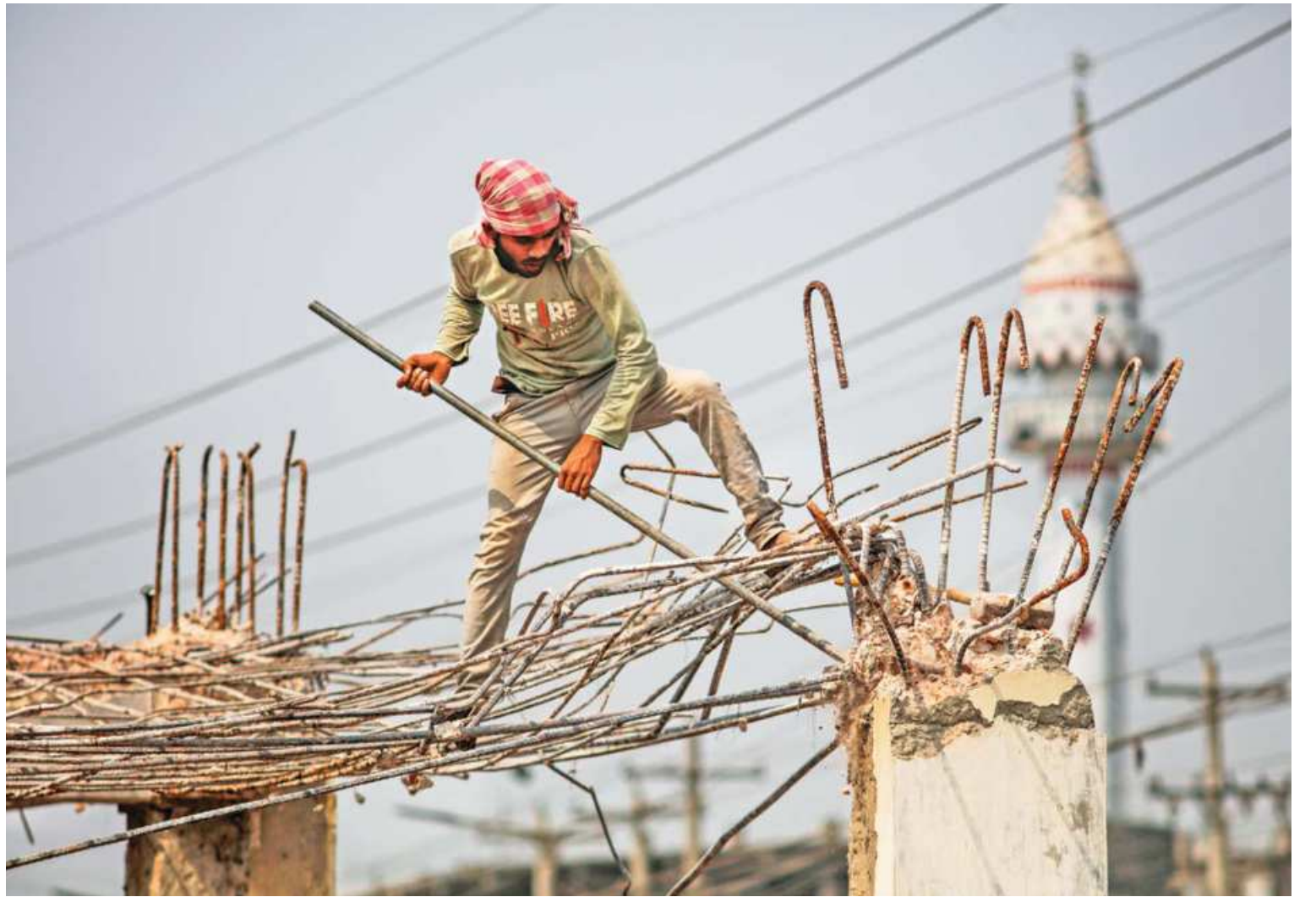
Without any safety gear, a construction worker demolishing an establishment in Aminbazar, on the outskirts of the capital, yesterday. He could fall and badly hurt himself.
