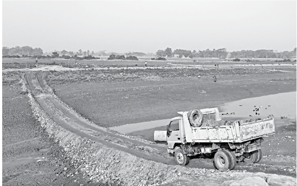
A truck driving down the road that was recently made by the owners of a brick kiln, across the Ubdakhali river in Kalmakanda upazila of Netrakona.
