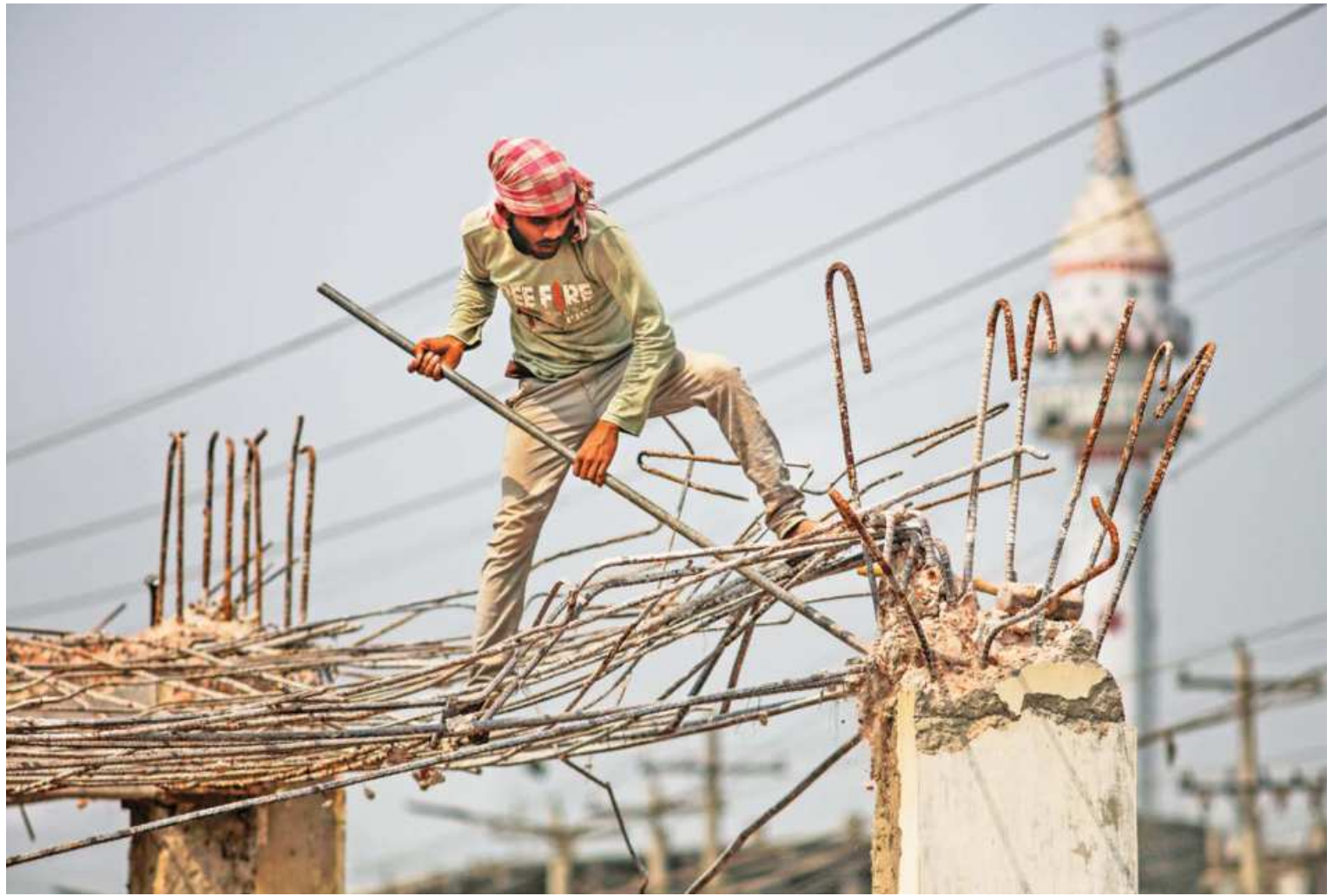
THINKING LITTLE BEFORE DOING ... Without any safety gear, a construction worker demolishing a building in Aminbazar, on the outskirts of the capital, yesterday. He is unaware that he is trying to get the rods he is standing on out. Many such buildings were recently torn down by their owners besides the Dhaka-Aricha highway to make way for a development project.
