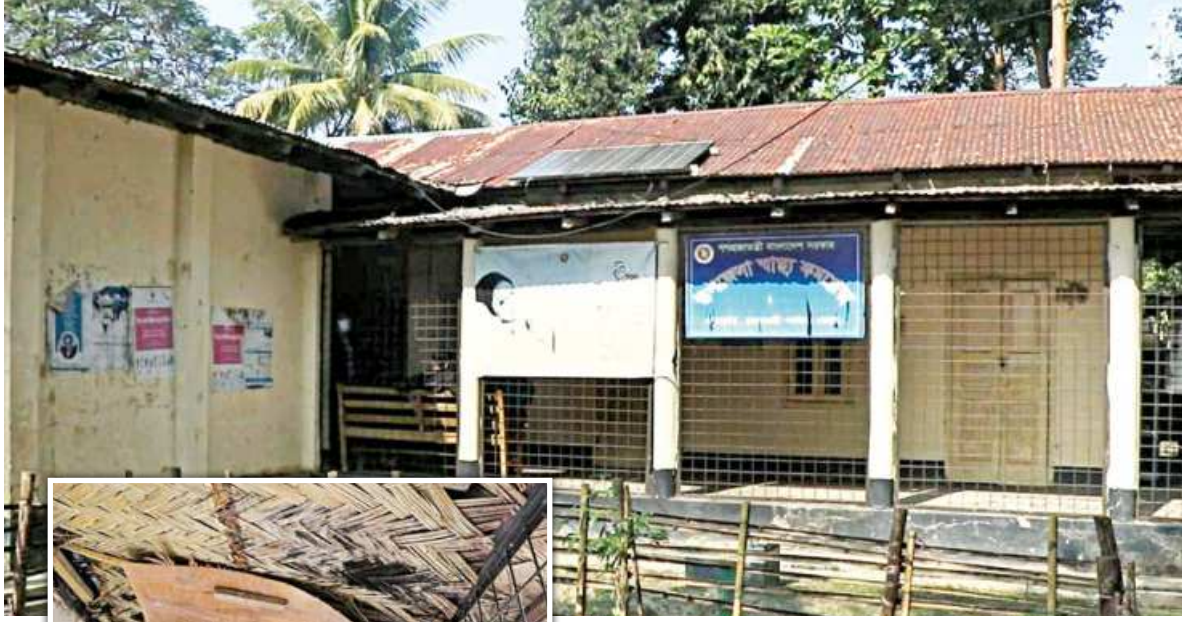
Jurachhari Upazila Health Complex in Rangamati. Inset, built in 1978, the health complex is yet to see any infrastructural development. The wall of that hospital is at risk of collapse any moment. PHOTO: STAR
