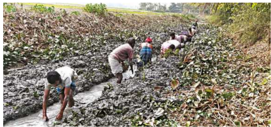
Local volunteers prepare a canal for re-excavation. The two-kilometre long Jauta-Naumala-Boga canal, in Patuakhali's Baulal upazila, has been dormant for around two decades.
