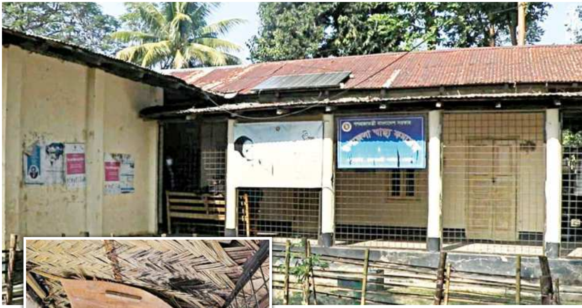
Jurachhari Upazila Health Complex in Rangamati. Inset, built in 1978, the health complex is yet to see any infrastructural development. The wall of that hospital is at risk of collapse any moment. PHOTO: STAR
