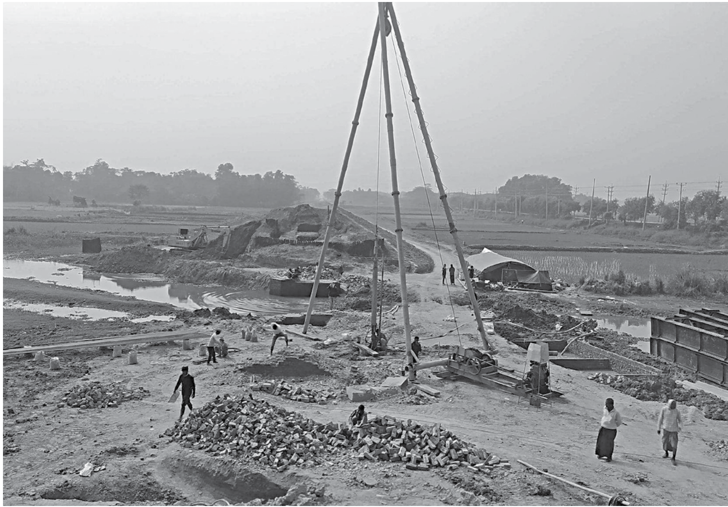
Due to lack of supervision of the contractor, only 30 percent of the Kulaura-Shahbajpur rail track rehabilitation work in Moulvibazar has been completed. However, the deadline for the rehabilitation work has expired in December last year.
