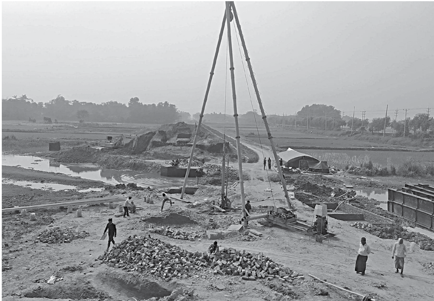
Due to lack of supervision of the contractor, only 30 percent of the Kulaura-Shahbajpur rail track rehabilitation work in Moulvibazar has been completed. However, the deadline for the rehabilitation work has expired in December last year.
