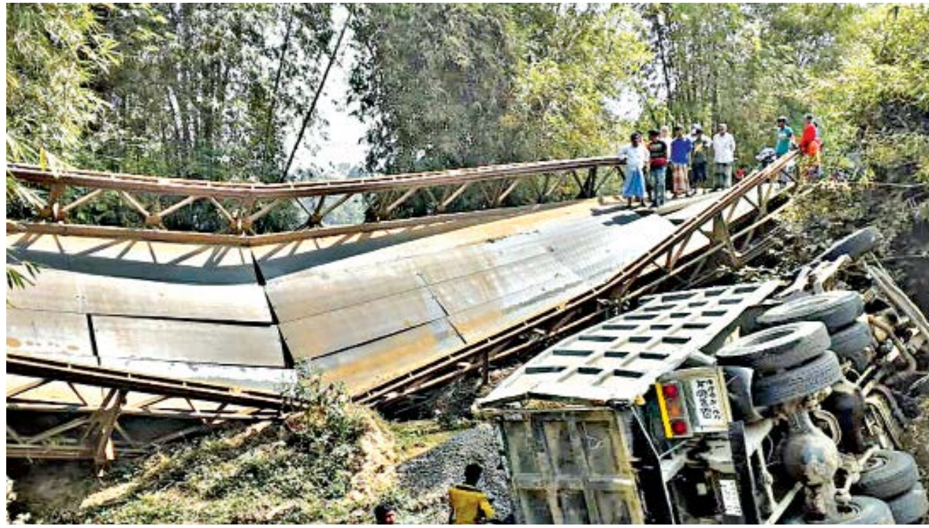
A Bailey bridge over a stream collapsed at Bangalhalia in Rangamati's Rajasthali unable to handle the load of a construction materials-laden truck that was crossing it on Thursday afternoon. Road communications between Bandarban and Rangamati remains snapped since, causing travellers of the two hill districts to suffer. Mosleh Uddin Chowdhury, executive engineer of Roads and Highways Department in Bandarban, said they started repairs but it would take around a week.
