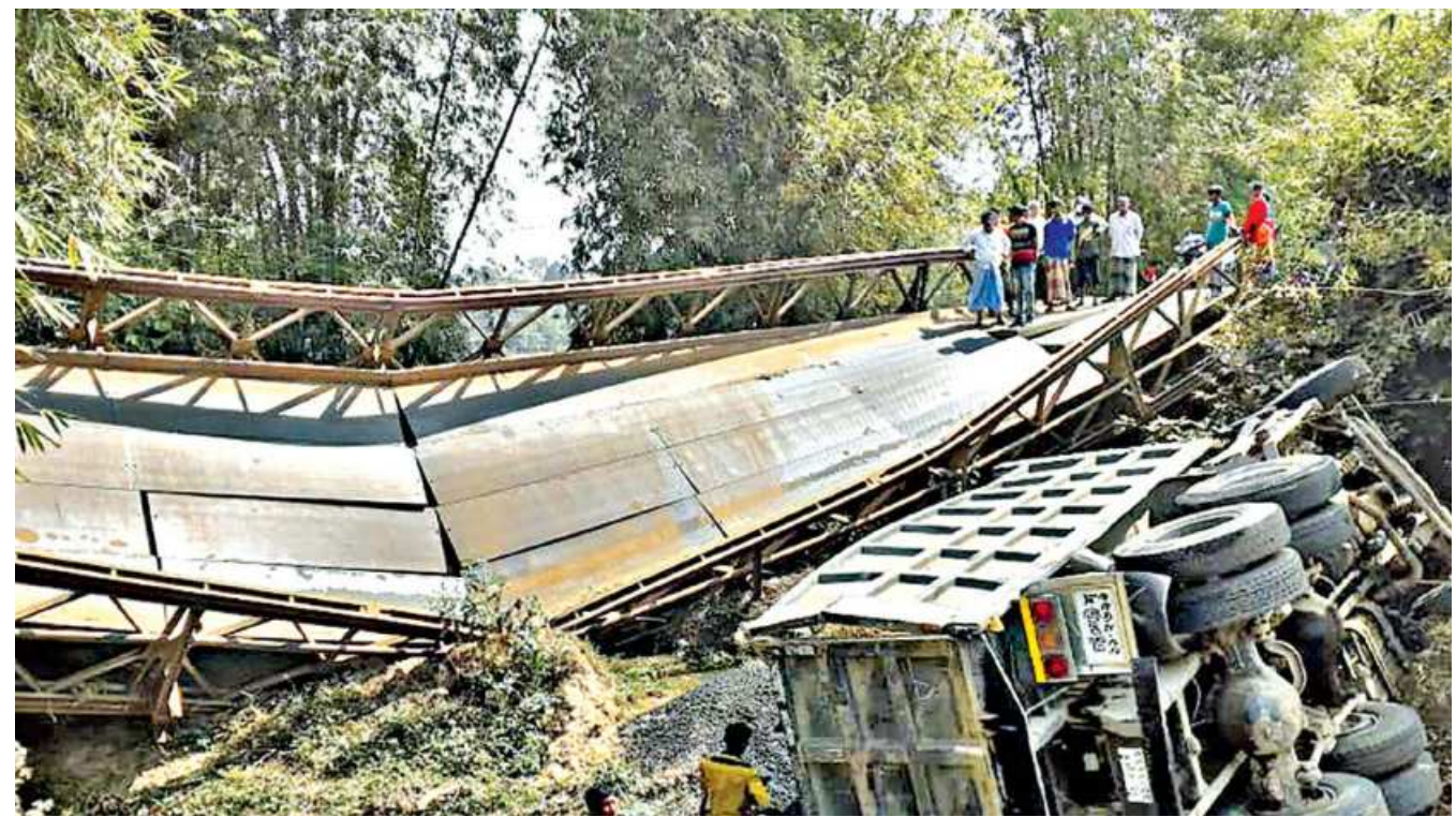
A Bailey bridge over a stream collapsed at Bangalhalia in Rangamati's Rajasthali unable to handle the load of a construction materials-laden truck that was crossing it on Thursday afternoon. Road communications between Bandarban and Rangamati remains snapped since, causing travellers of the two hill districts to suffer. Mosleh Uddin Chowdhury, executive engineer of Roads and Highways Department in Bandarban, said they started repairs but it would take around a week.
