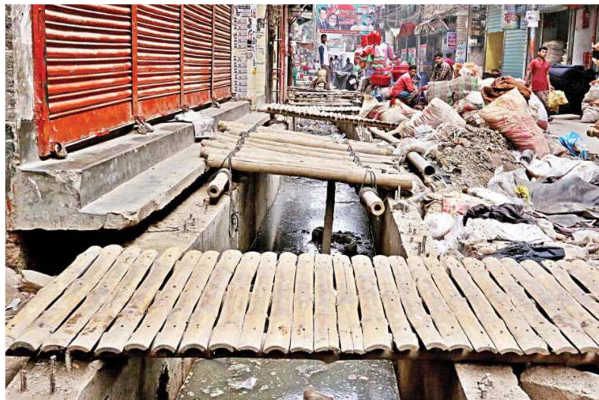
Development work of drainage in Old Dhaka's Aga Masih Lane has been going on at a snail's pace for around two months now, locals of the area claim. They allege the contractor has employed too few workers, which results in the continuing suffering in the busy area. This photo was taken yesterday.
