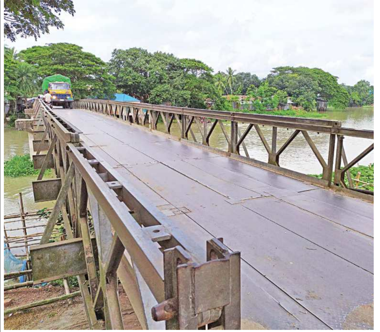
Faridpur Roads and Highways Department (RHD) waiting for approval from the authorities concerned to replace this iron structured bailey bridge in Nagarkanda upazila with a concrete one. The 18-feet-long and only 10-feet-wide bridge over the Kumar river on Faridpur-Muksudpur road often sees huge traffic jam on the busy road as vehicles from either side cannot ply the bridge at a time due to its narrowness. Moreover, the dilapidated bridge, which awaits renovation for long, has already turn risky for its users.
