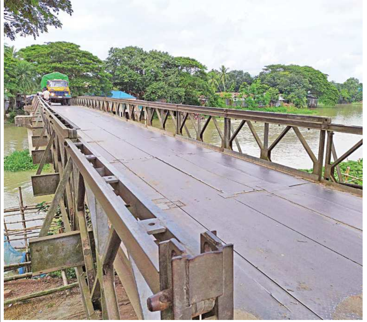
Faridpur Roads and Highways Department (RHD) waiting for approval from the authorities concerned to replace this iron structured bailey bridge in Nagarkanda upazila with a concrete one. The 18-feet-long and only 10-feet-wide bridge over the Kumar river on Faridpur-Muksudpur road often sees huge traffic jam on the busy road as vehicles from either side cannot ply the bridge at a time due to its narrowness. Moreover, the dilapidated bridge, which awaits renovation for long, has already turn risky for its users.
