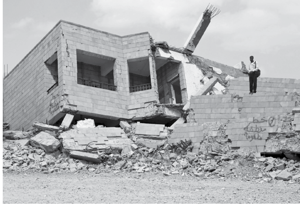
A Yemeni student stands on top of the debris of a school in March 2019, which was damaged following a Saudi-led coalition air strike.
