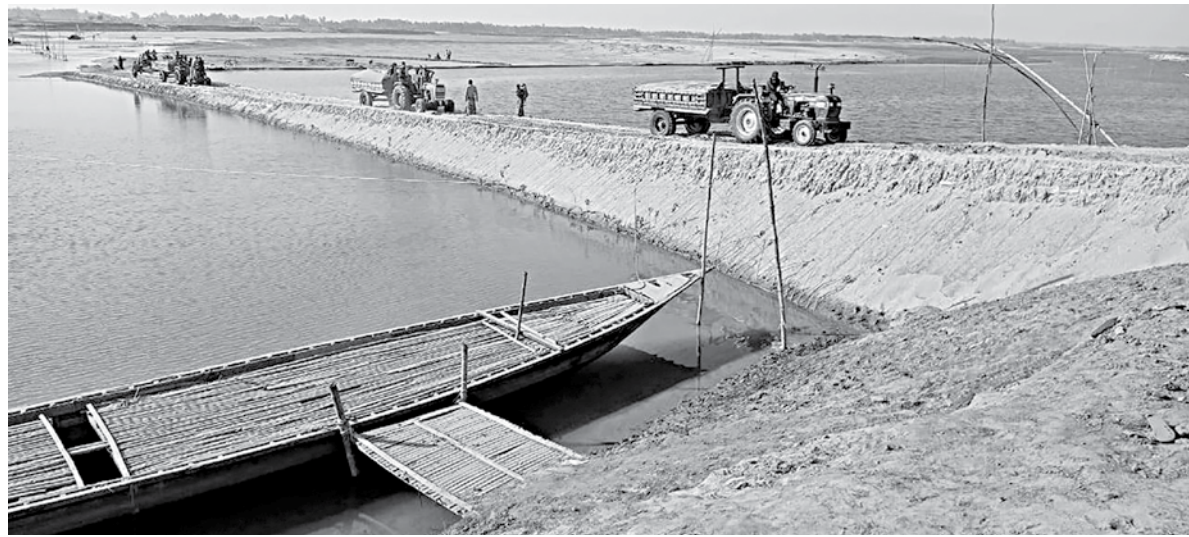
The sandy road has been built on the Brahmaputra river bed in Kartimari Nou Ghat area of Kurigram's Roimari upazila for carrying sand. Illegal sand lifting from the river in the area, posing a threat to the nearby embankment.
