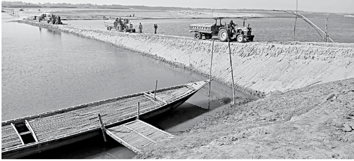
The sandy road has been built on the Brahmaputra river bed in Kartimari Nou Ghat area of Kurigram's Roimari upazila for carrying sand. Illegal sand lifting from the river in the area, posing a threat to the nearby embankment.
