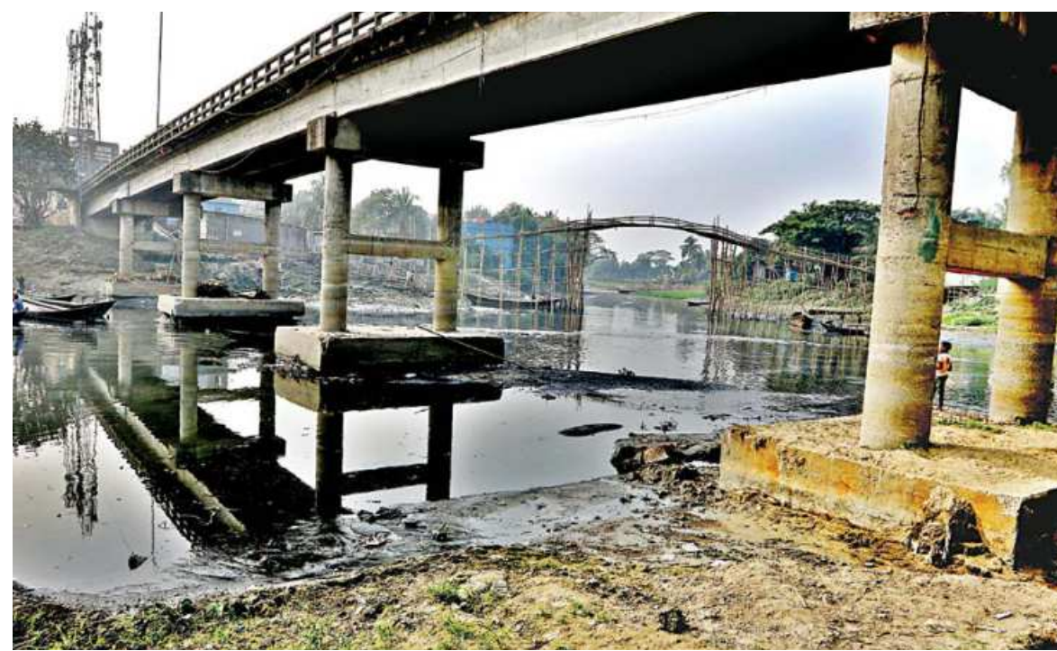
Pile caps and piers of the Trimohoni bridge on the Balu river are visible as the water body has dried up in the capital's Khilgaon area. The water has also become dark due to pollution. The photo was taken recently.
