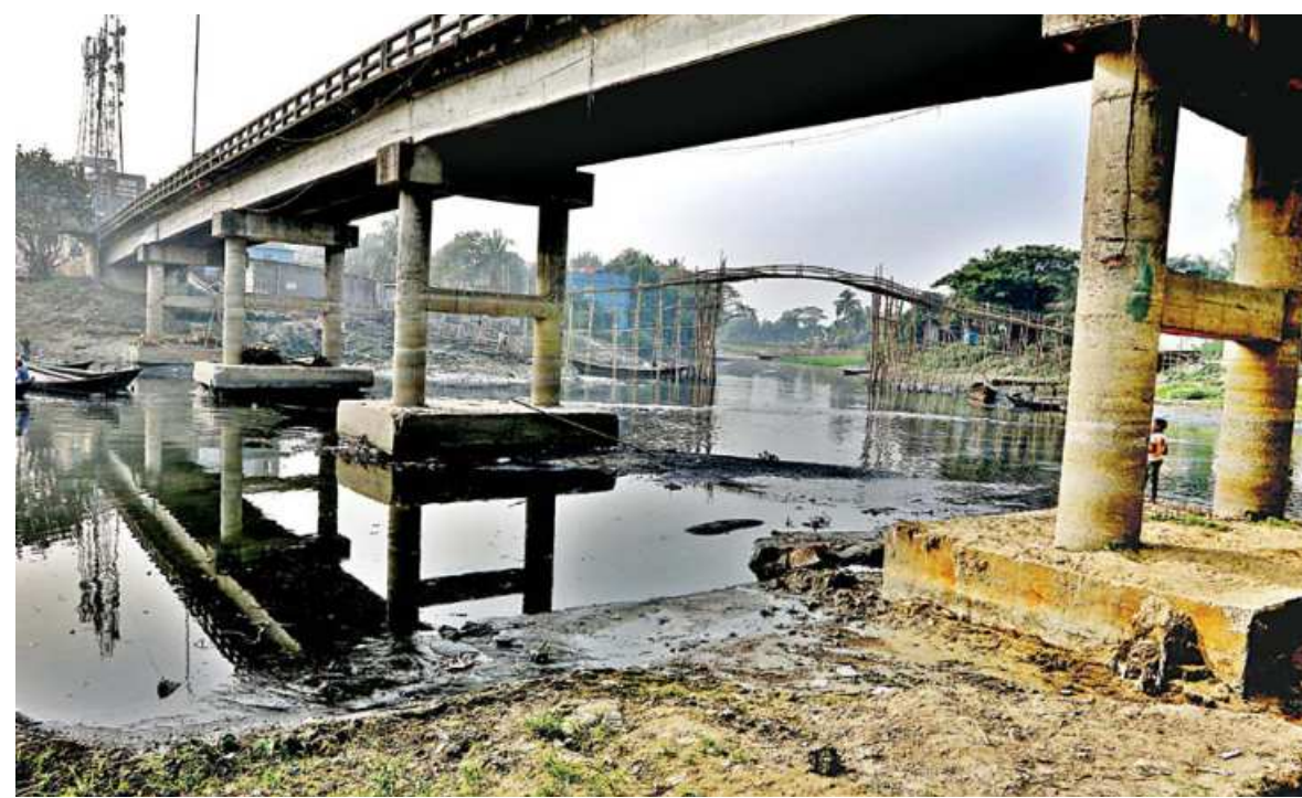
Pile caps and piers of the Trimohoni bridge on the Balu river are visible as the water body has dried up in the capital's Khilgaon area. The water has also become dark due to pollution. The photo was taken recently.
