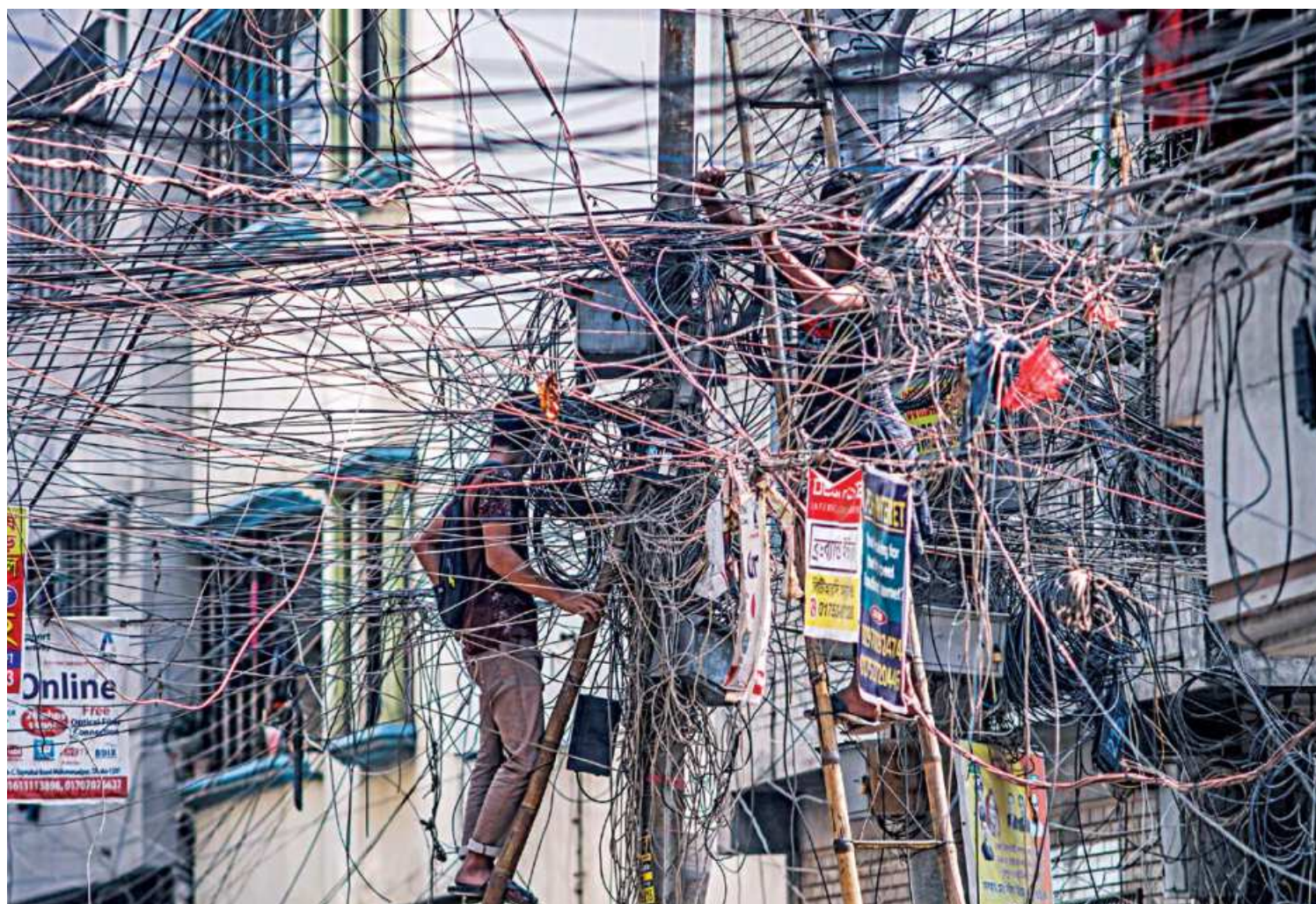
Workers set up unplanned fiber optic and dish cables without safety gear. Various service providers are making their staffers do such work without necessary precaution, which is ultimately making them risk their lives in case of short-circuits. The photo was taken yesterday at Mohammadpur's Haji Chinu Mia Road.
