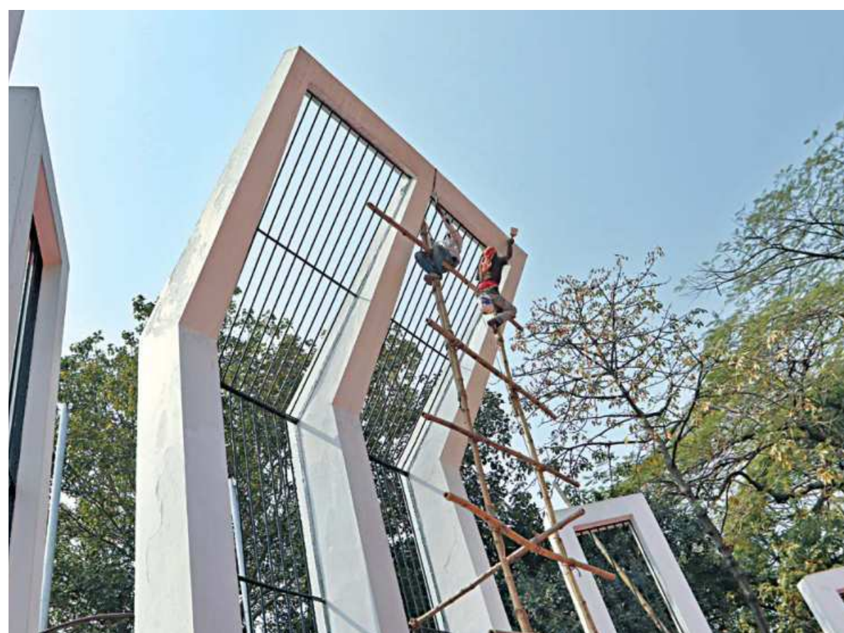
Two workers repaint the Central Shaheed Minar in the capital, with less than two weeks to go for International Mother Language Day. However, the flimsy bamboo structure used instead of scaffolding for the work has left them perched in a precarious and unsafe position at a dangerous height. The photo was taken yesterday.
