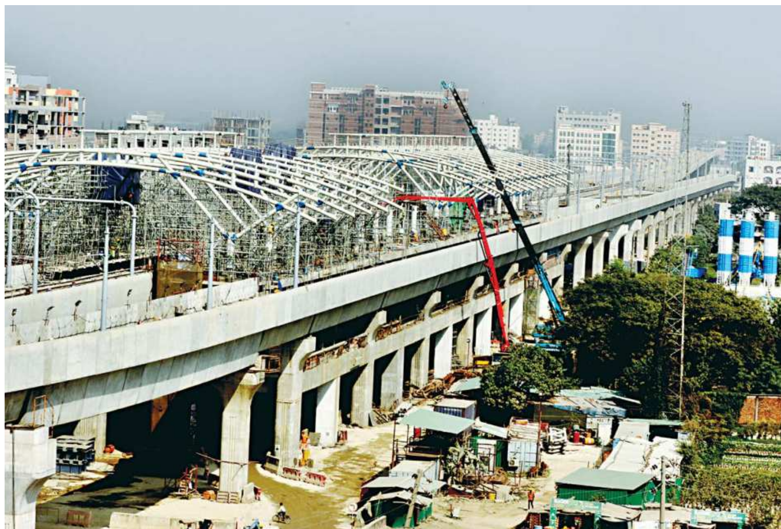
A view of the Metro Rail station at Uttara's Diyabari in the capital. Construction work of the station is almost complete and it has already become a landmark in the area. The Mass Rapid Transit-6 line starts from this station in Diyabari. The photo was taken yesterday.
