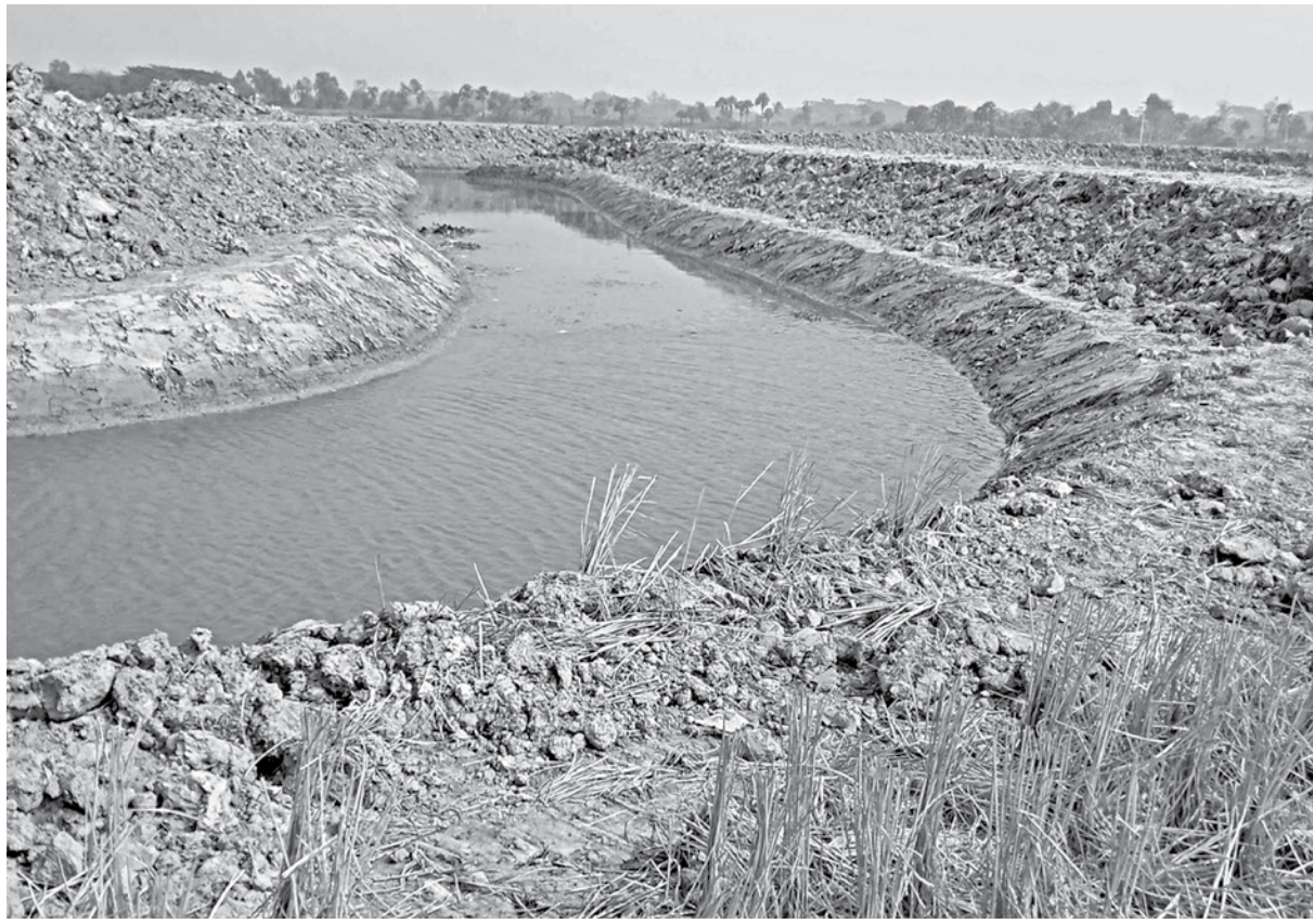
One of the re-excavated canals that became a source of hope for farmers in three villages of Patuakhali's Kalapara upazila. The photo was taken recently.
