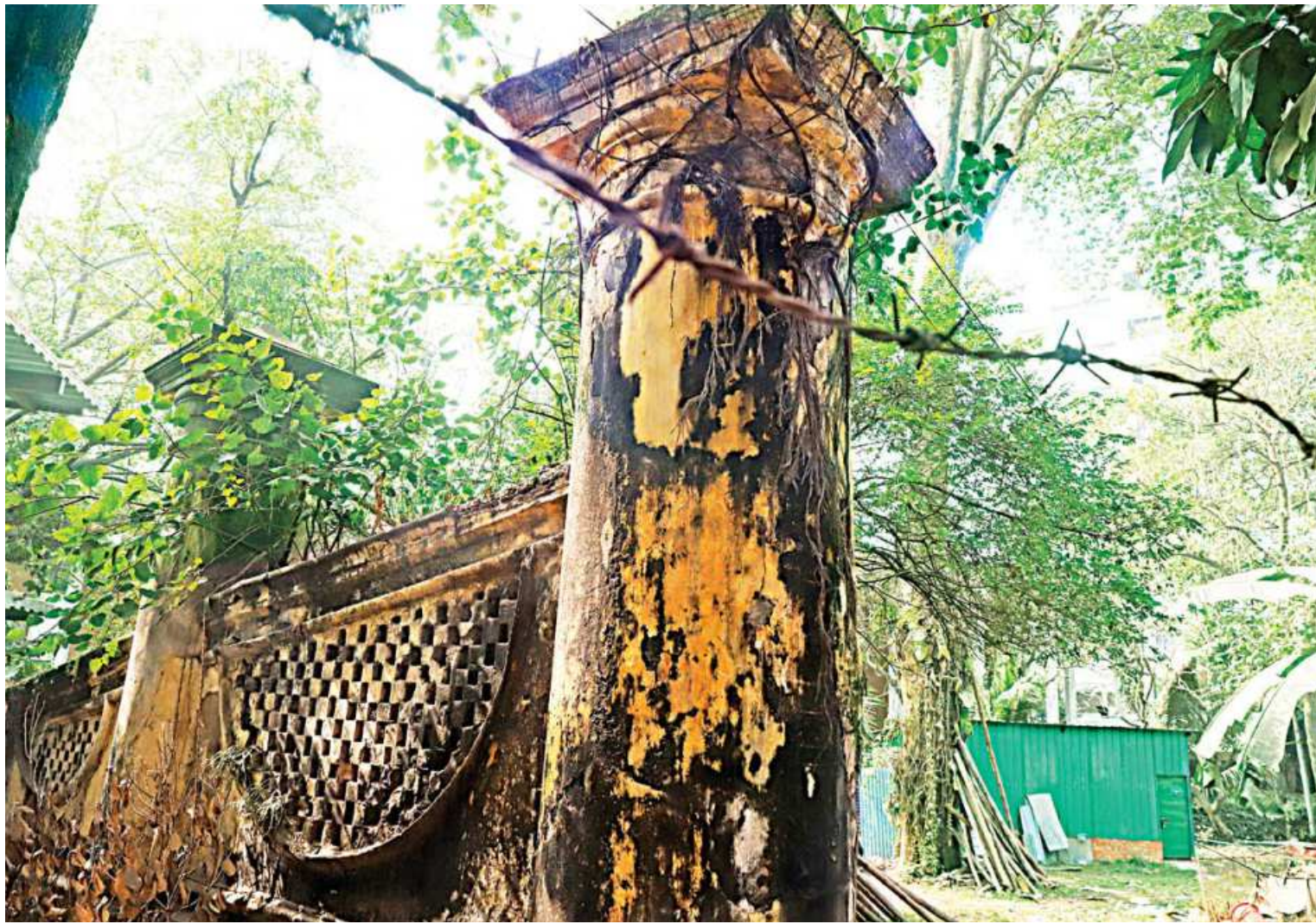
Resembling remnants of an abandoned structure, this portion of Dhaka Gate, an iconic part of Dhaka's Mughal history dating back over 400 years, lies in shambles. Popularly believed to have been erected by Subedar Mir Jumla II in the mid-17th century as the northern entry point to Dhaka, after its reestablishment as the capital of Bengal. It is thought to have been rebuilt in 1825 by British Magistrate Charles Dawes. However, little appears to have been done to preserve this piece of history. The photo was taken recently.
