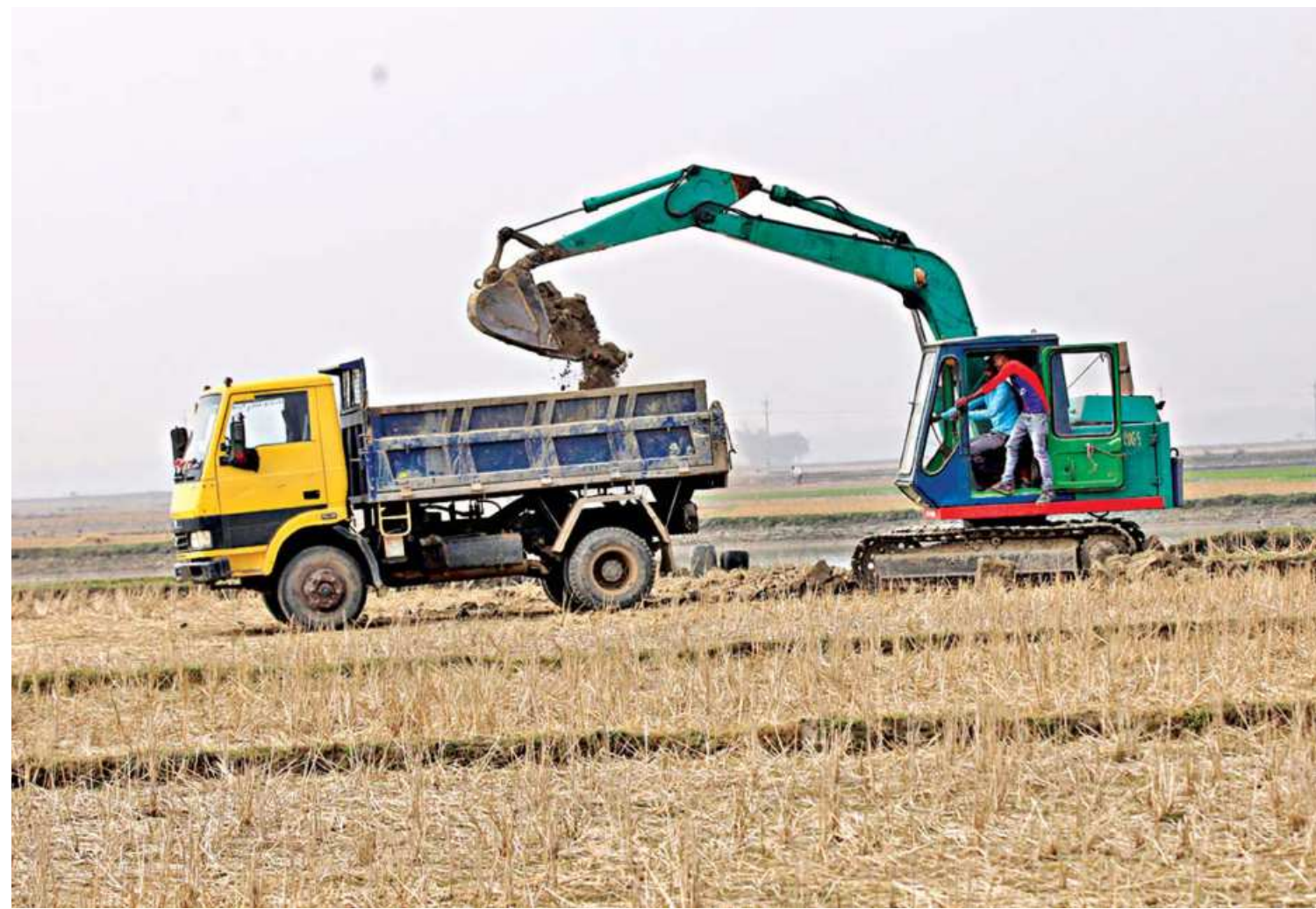
The top soil of croplands are being cut and taken away in Sylhet's Companyganj upazila. Locally influential people collect the soil in exchange of a minimal amount from farmers. The soil is then sold to brick kilns at a much higher price. This process destroys alluvium of the fields, eventually affecting the farmers and the economy. The photo was taken recently.
