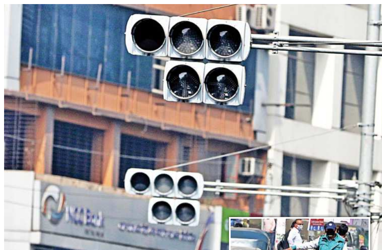
Traffic lights at Gulshan-1, a major intersection in one of the most upscale neighbourhoods of the capital, remain out of order, as traffic police are left with the task to manage the busy thoroughfare with hand signals, inset. The photos were taken yesterday.
