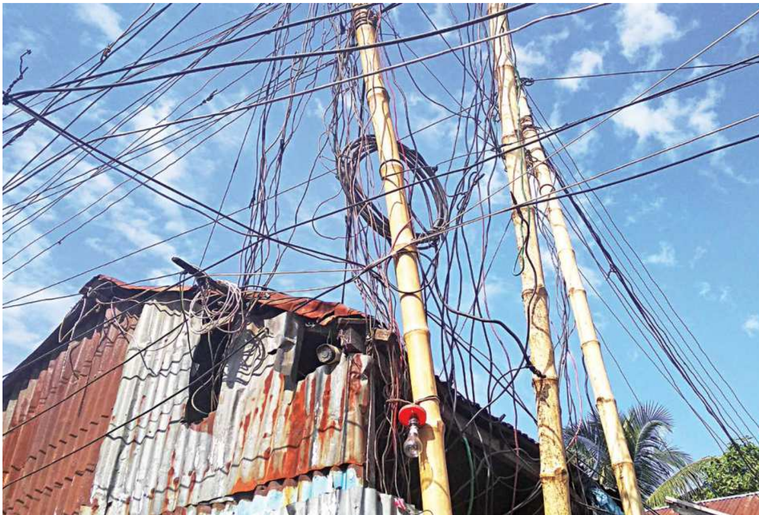
A tangle of electrical wires from a small tin shed crisscrossing in haphazard fashion in the capital's Karail slum. A main electrical line was seen going into the shed, and all these wires were presumably connected to it to provide electricity throughout the slum. This causes a risk of fire in the densely populated area.
