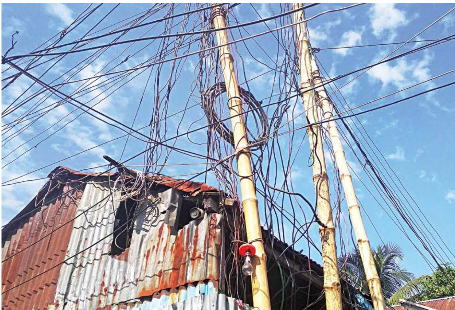
A tangle of electrical wires from a small tin shed crisscrossing in haphazard fashion in the capital's Karail slum. A main electrical line was seen going into the shed, and all these wires were presumably connected to it to provide electricity throughout the slum. This causes a risk of fire in the densely populated area.
