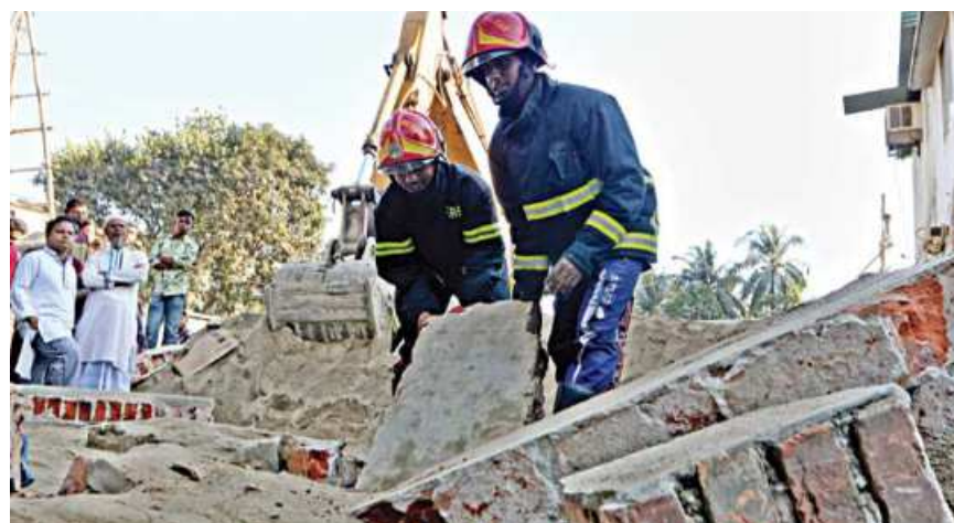
A Power Development Board driver and another person were killed after a wall collapsed on them at the Port City's Debarpar yesterday afternoon. According to fire service officials, the accident took place when an excavator hit the wall adjacent to the sand it was removing.
