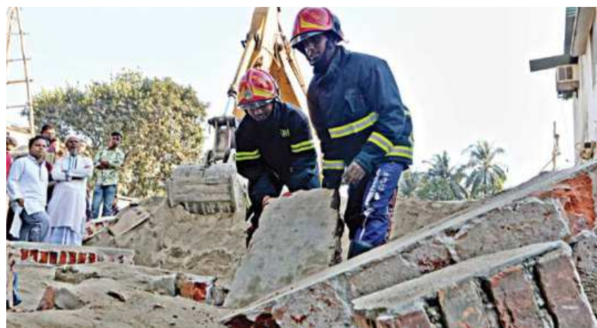
A Power Development Board driver and another person were killed after a wall collapsed on them at the Port City's Debarpar yesterday afternoon. According to fire service officials, the accident took place when an excavator hit the wall adjacent to the sand it was removing.
