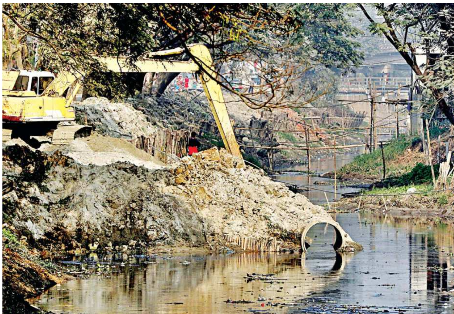
Dhaka South City Corporation conducts a drive on Jirani canal in the capital's Trimohoni area to protect it from encroachment and improve its navigability. Dhaka Water Supply and Sewerage Authority recently handed over the canal to the corporation. The photo was taken yesterday.
