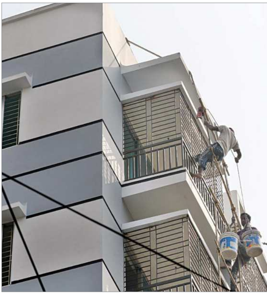
Workers hang off of a flimsy self-improvised harness to complete the paint job at this building in Razabazar yesterday, just another day of extremely unsafe work conditions for labourers in Dhaka.
