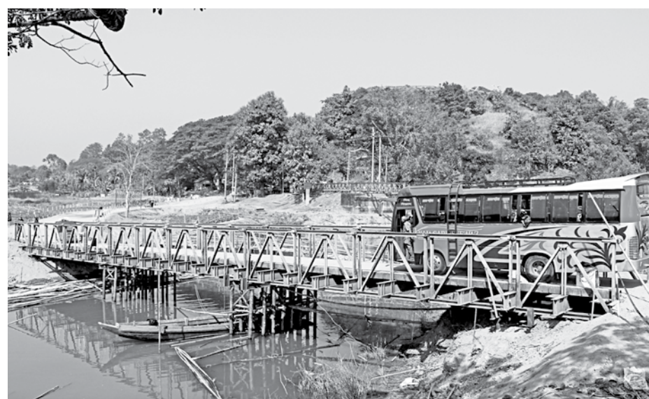
After nearly two weeks of suspension road communication through Rangamati-Khagrachhari Link Road resumes yesterday. The Roads and Highways Department and Bangladesh Army 20 ECB jointly constructed a 140-foot-long temporary Bailey bridge next to the collapsed one. On January 12, the bridge collapsed when a stone-laden truck was crossing Boro Mohapurom Chhara, leaving three people killed.
