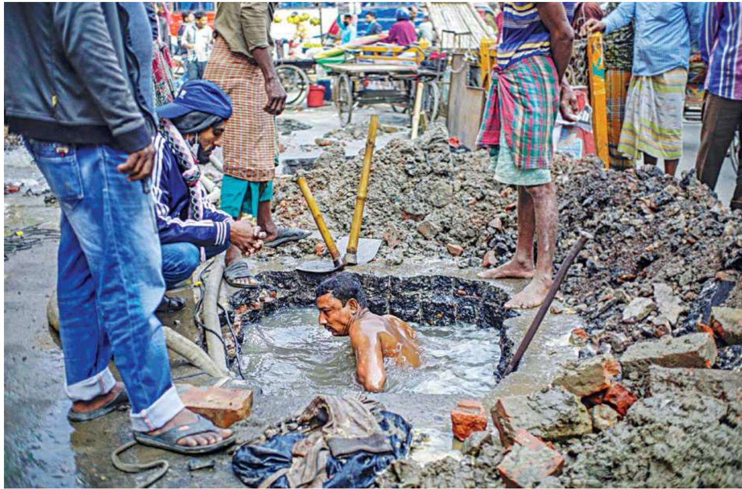
A worker of Dhaka Wasa braves the cold to get down into the water inside a pothole in the capital's Nazirabazar, Bongshal yesterday. While authorities responsible for maintaining the city's utility services often get flak for negligence in serving citizens, such commitment of field-level employees is certainly heartening. The photo was taken on Saturday.
