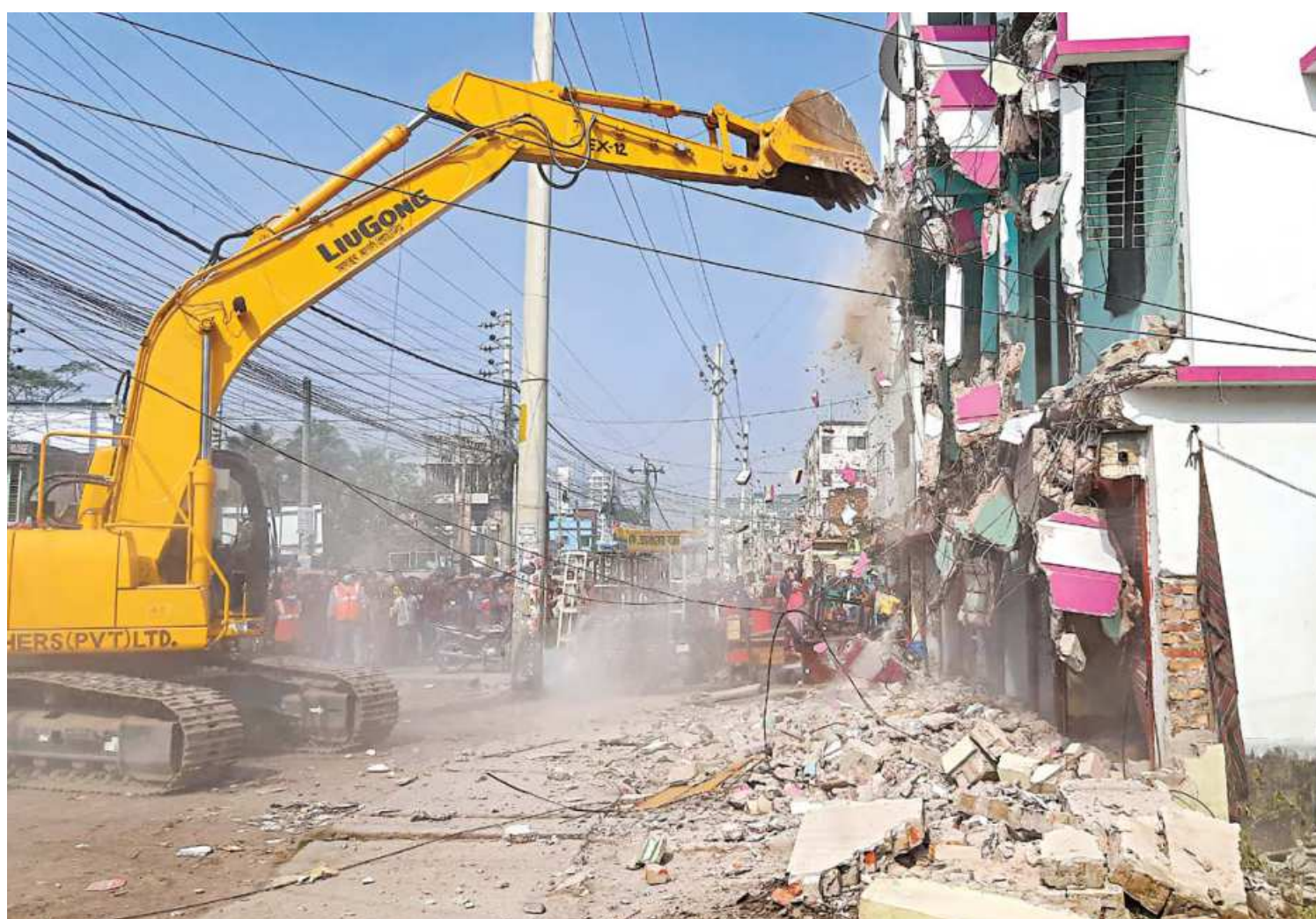
Roads and Highways Department has been demolishing illegal structures on Khulna city's Sher-e-Bangla Road for a week, to turn the two-lane road into a four-lane one. Till yesterday, around 70 buildings were demolished during the ongoing eviction drive. The photo was taken from Amtola intersection yesterday.
