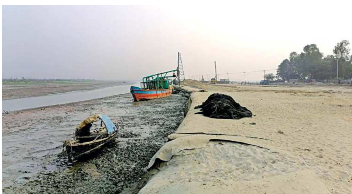
The portion of the Kohelia river in Moheshkhali's Matarbari union is in a sorry state after an under-construction four-lane highway began encroaching upon the once might water body five years ago. The photo was taken recently.
