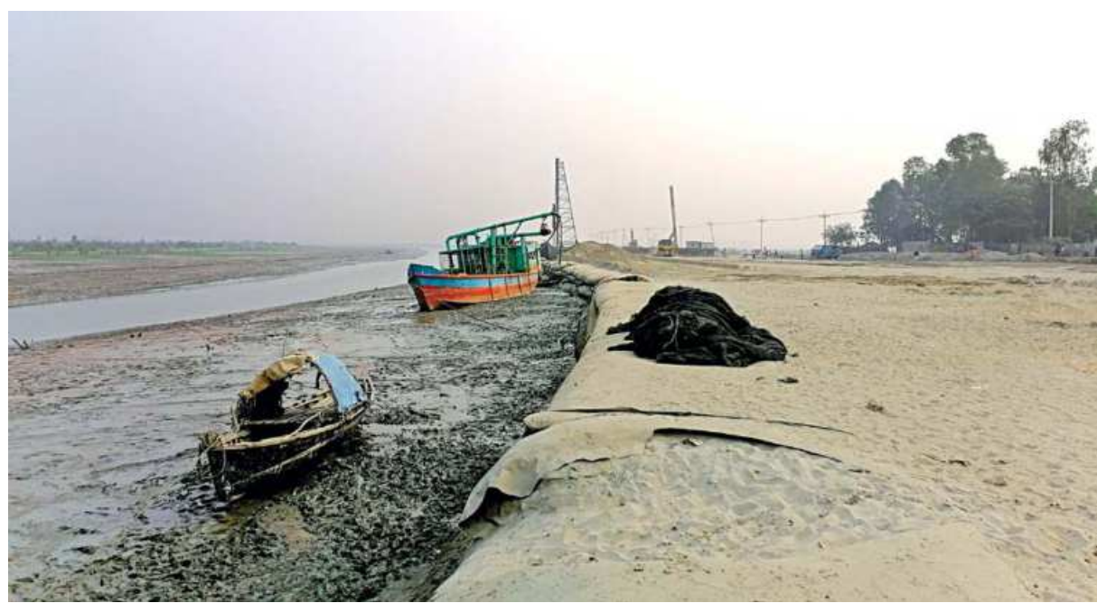
This portion of the Kohelia river in Moheshkhali's Matarbari union is in a sorry state after an under-construction four-lane highway began encroaching upon the once mighty river five years ago. The photo was taken recently.
