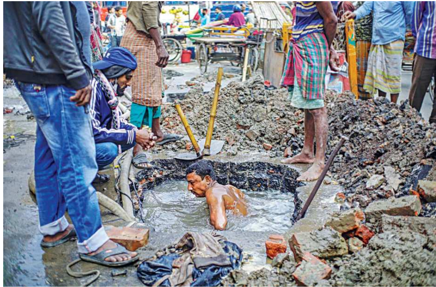
A worker of Dhaka Wasa braves the cold to get down into the water inside a pothole in the capital's Nazirabazar, Bongshal yesterday. While authorities responsible for maintaining the city's utility services often get flak for negligence in serving citizens, such commitment of field-level employees is certainly heartening. The photo was taken on Saturday.
