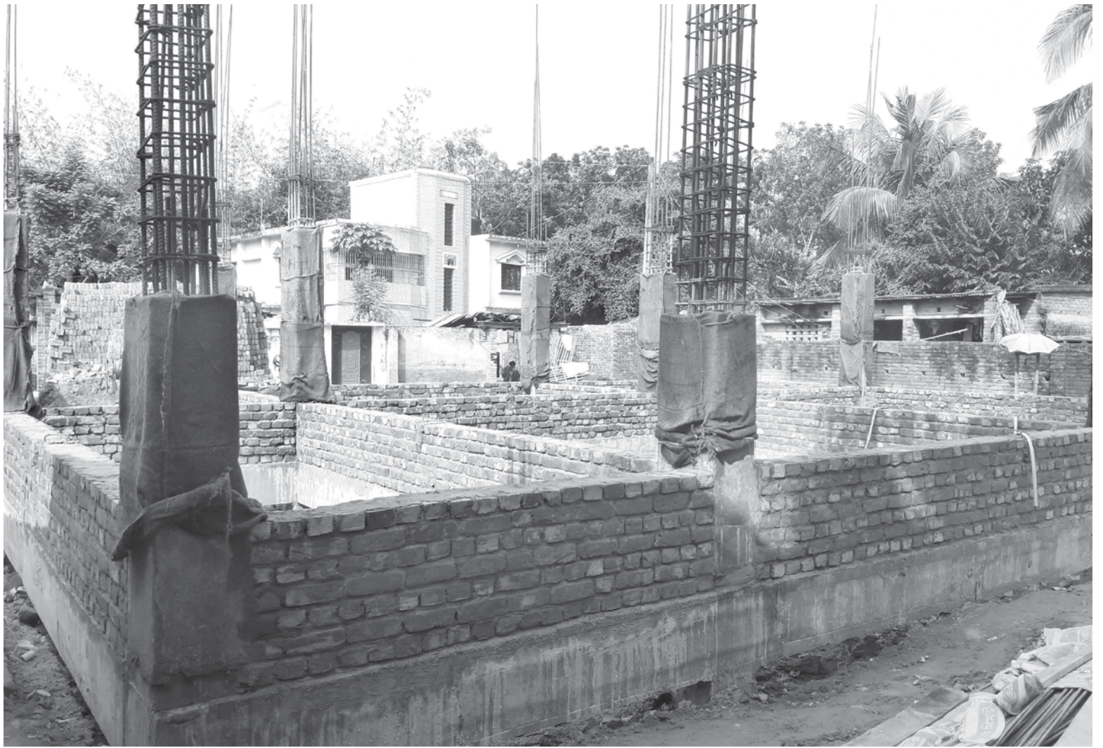
The work to reconstruct the Birshreshtha Hamidur Rahman memorial building, in Khordakhalishpur village of Jhenidah's Moheshpur upazila, is going on in full swing. The photo was taken recently.
