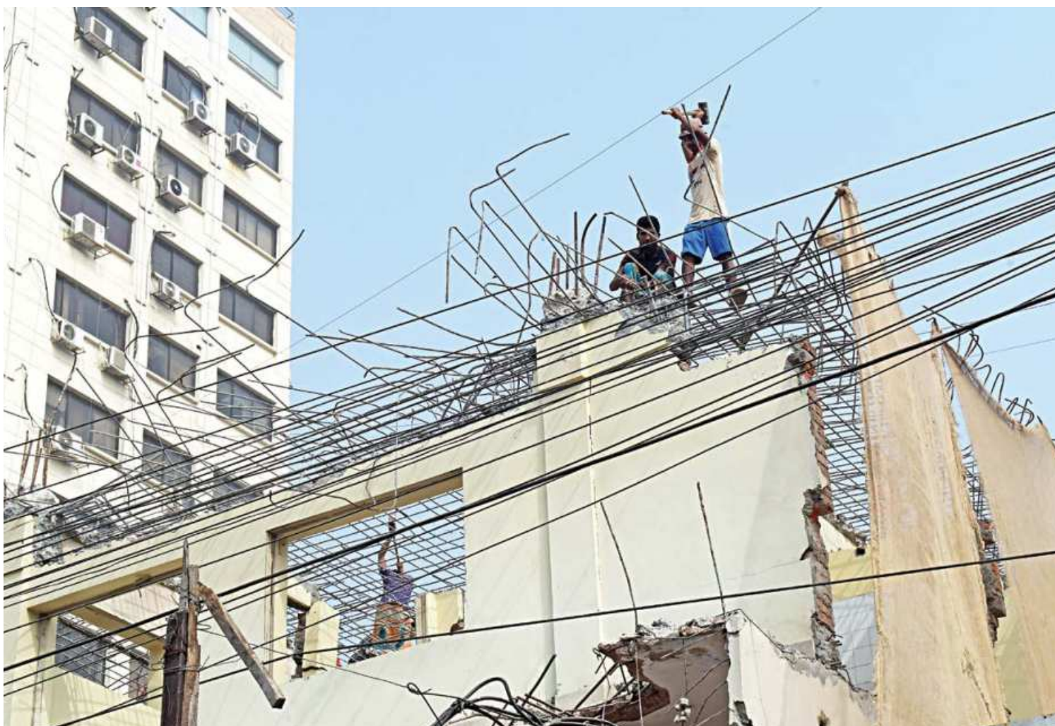
Workers without any safety equipment knock down an old building in the capital's Farmgate area. Many workers die and suffer serious injuries because of such flagrant disregard for safety. The photo was taken on Thursday.
