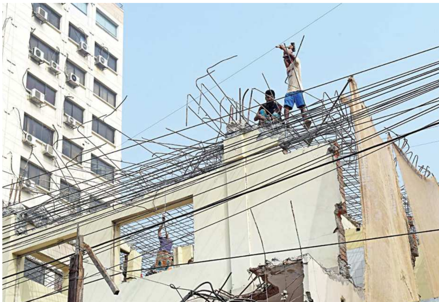
Workers without any safety equipment knock down an old building in the capital's Farmgate area. Many workers die and suffer serious injuries because of such flagrant disregard for safety. The photo was taken on Thursday.
