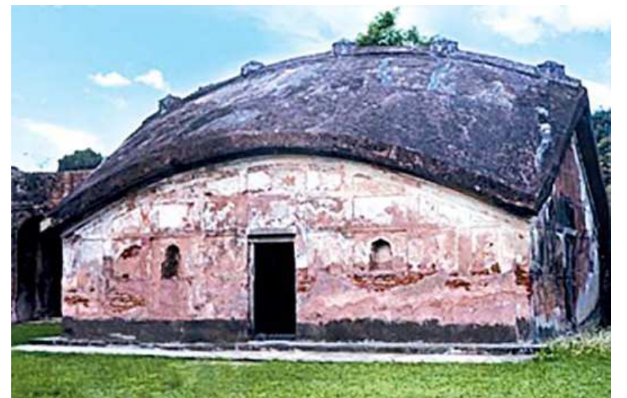
Fath Khan's Tomb, Gaur, West Bengal. It was built in imitation of a vernacular do-chala hut.
