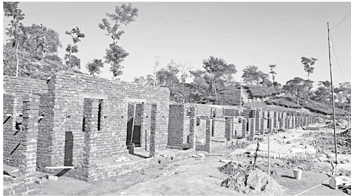
Houses for the homeless being built right at the bottom of slopes of hillocks, in Bishamani area of Srimangal upazila in Moulvibazar. The photo was taken recently.
