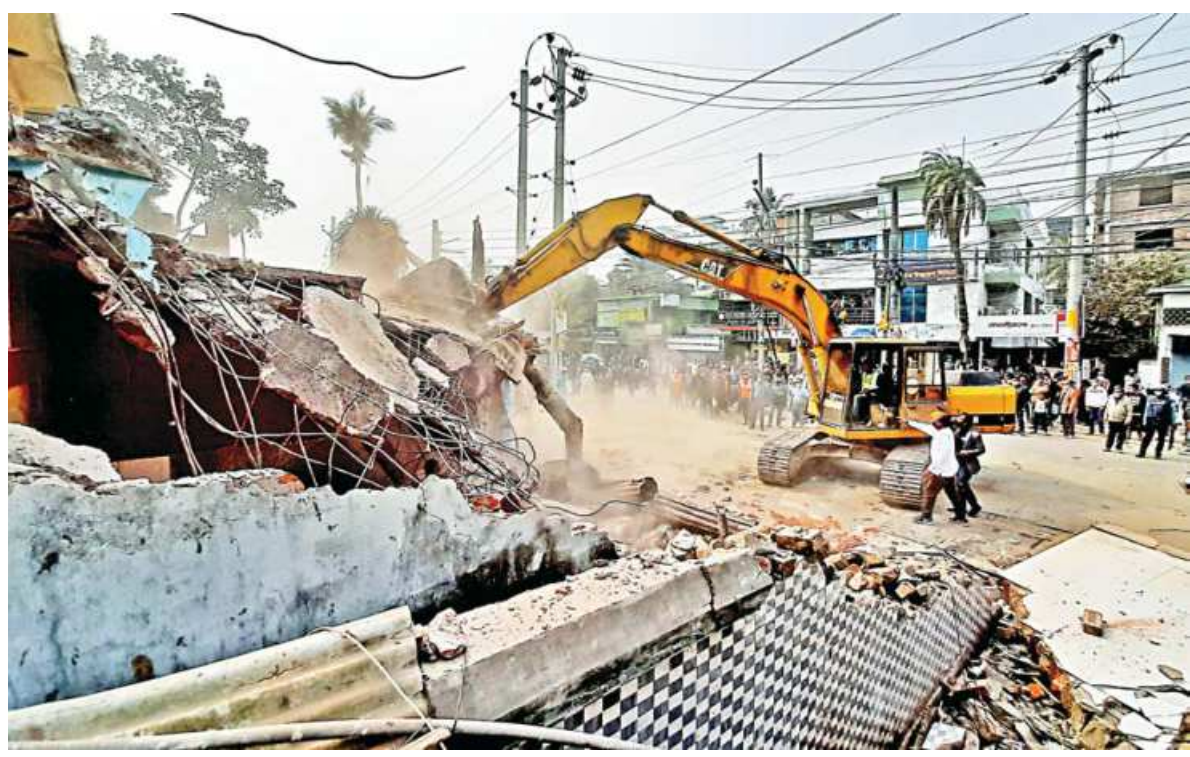
A crane demolishing a structure in Khulna's Moylapota area. The roads and highway department, with assistance from the Khulna City Corporation, conducted the drive to demolish structures that had encroached upon the road, which will be turned into a four-lane highway. The photo was taken around 11:30am yesterday.
