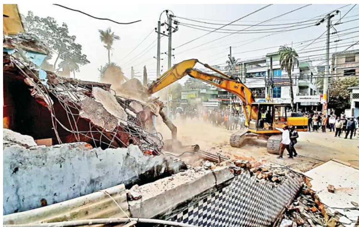
An excavator demolishing a structure in Khulna's Moylapota area. The roads and highway department, with assistance from the Khulna City Corporation, conducted the drive to demolish structures that had encroached upon the road, which will be turned into a four-lane highway. The photo was taken around 11:30am yesterday.
