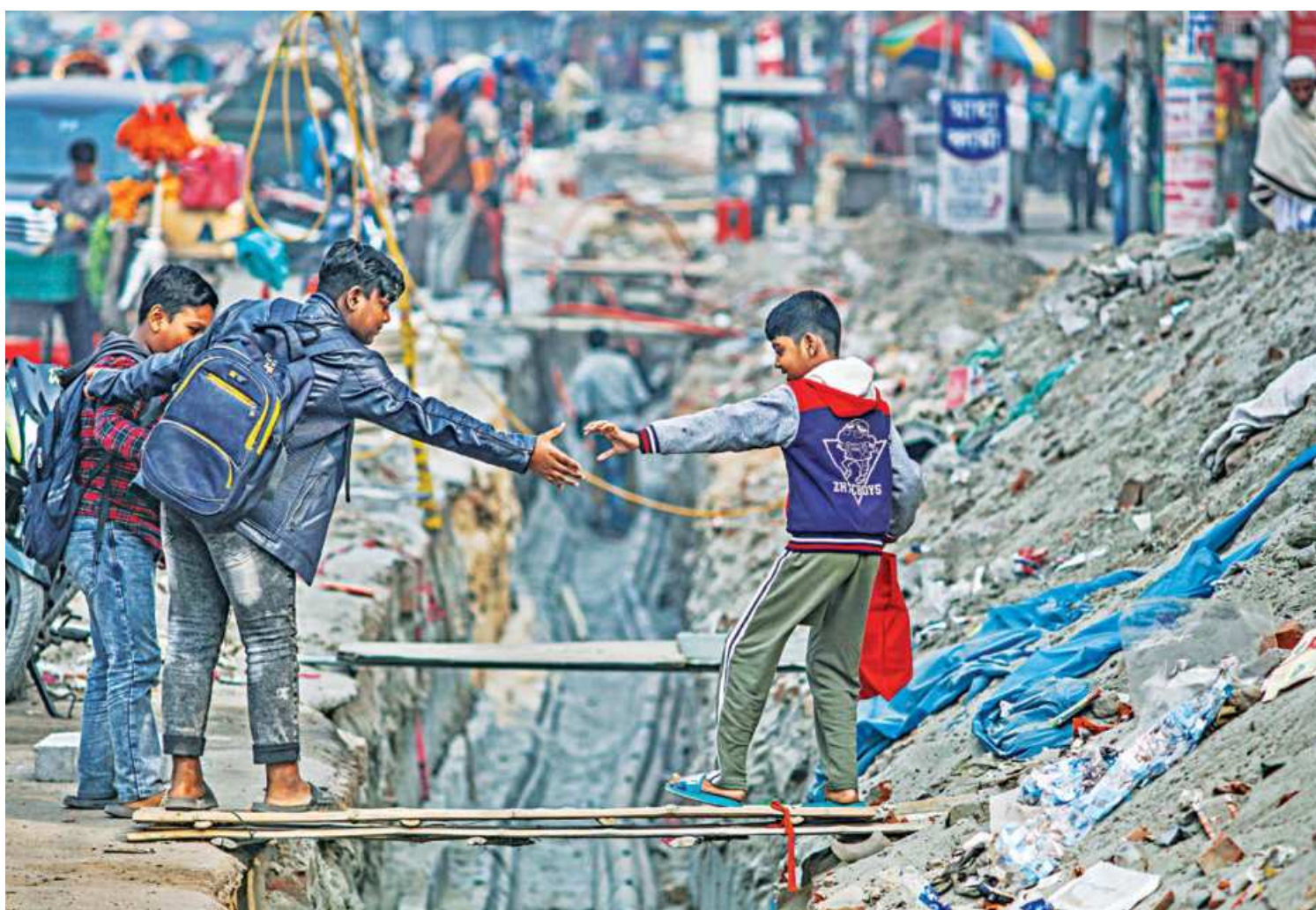
A young boy reaches out for help as he embarks on a balancing act to cross the deep trench by walking across on two narrow planks tied together to form a makeshift, flimsy footbridge. The Dhaka Power Distribution Company dug the trench along the road from the capital's Mohammadpur bus stand towards Bosila in order to lay high voltage power lines. The photo was taken at noon yesterday.
