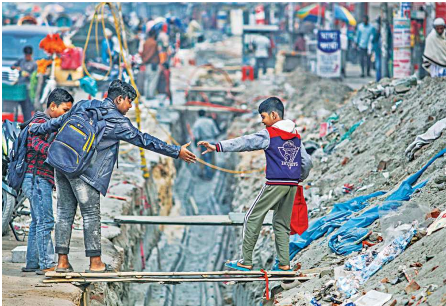
A young boy reaches out for help as he embarks on a balancing act to cross the deep trench by walking across on two narrow planks tied together to form a makeshift, flimsy footbridge. The Dhaka Power Distribution Company dug the trench along the road from Mohammadpur bus stand towards Bosila in the capital in order to lay high voltage power lines. The photo was taken at noon yesterday.
