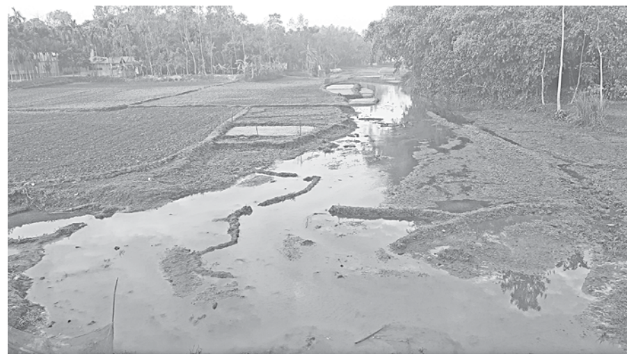
The LGED claims to have excavated this canal, in Charali Beel area of Aditmari upazila in Lalmonirhat, at a cost of Tk 45 lakh. But at places, there is only knee-deep water in it. The photo was taken recently.
