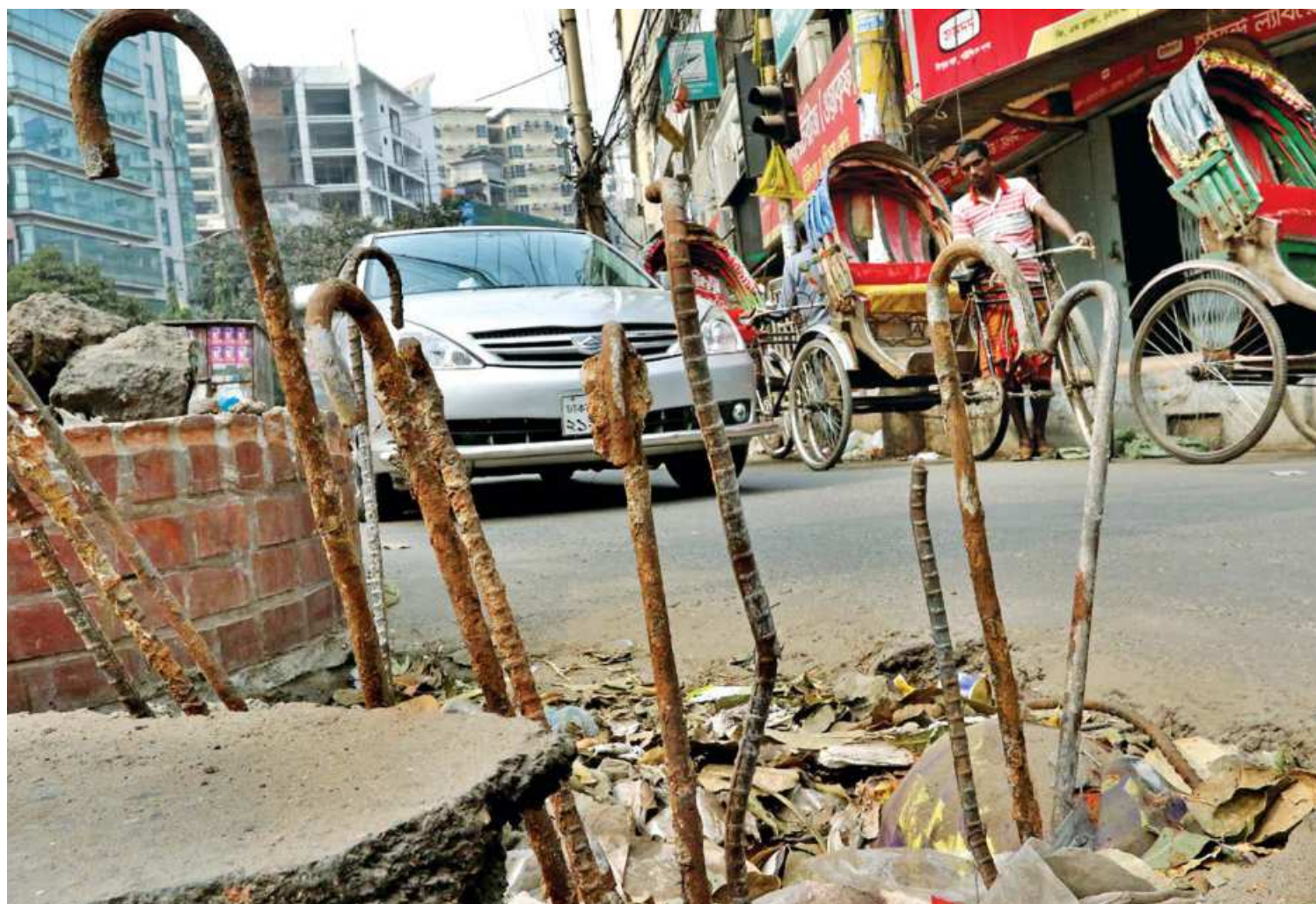
Rods sticking out of a manhole on the side of a road at the north-west corner of the Panthapath intersection in the capital. According to locals, the cover of the manhole had broken around a month ago and people had bent its rods outward to ward off vehicles. However, contrary to that purpose, the rods pose a danger to vehicles which pass perilously close. The photo was taken recently.
