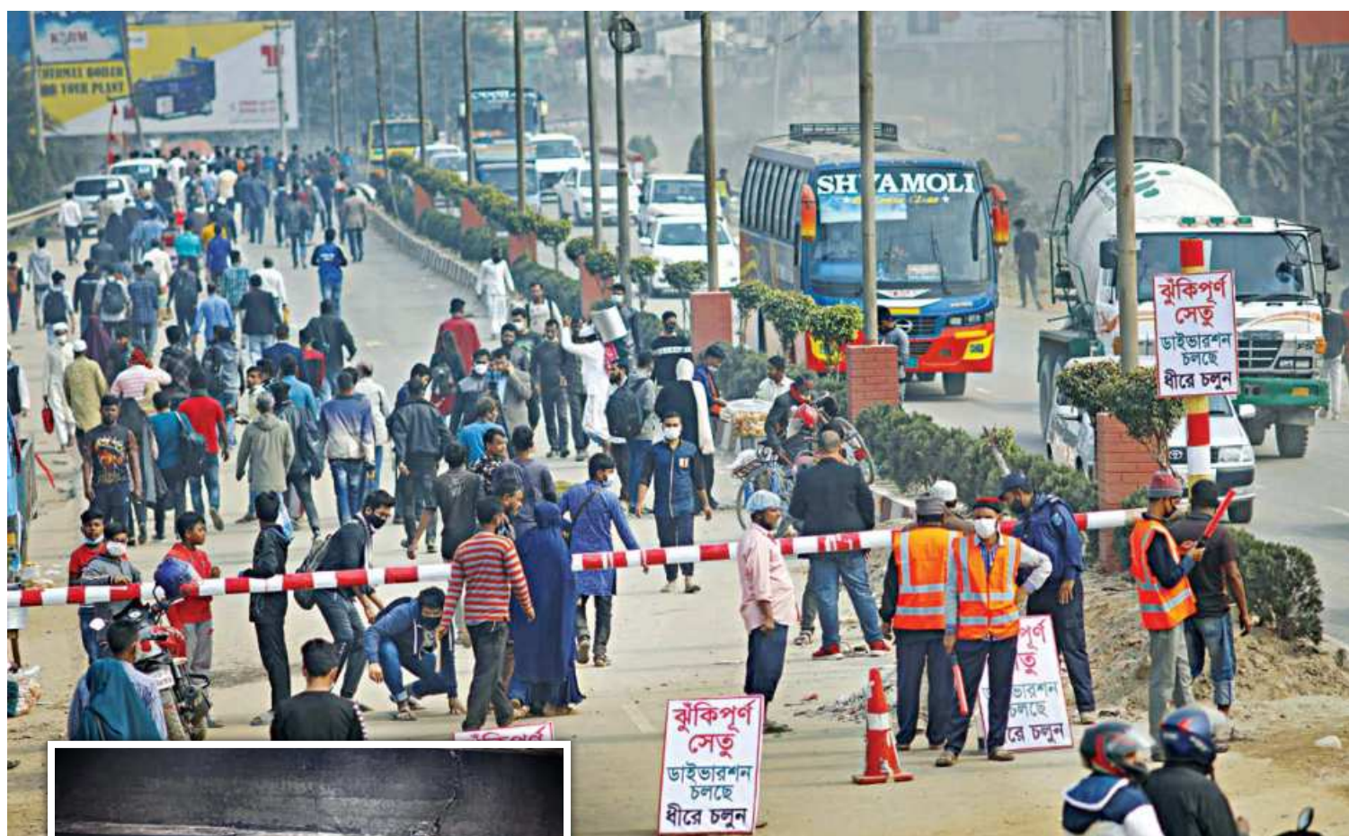
The authorities closed one side of Salehpur bridge on Dhaka-Aricha highway near Aminbazar after cracks, inset, were detected on a girder Wednesday afternoon. It created huge tailbacks on one of the busiest highways in the country throughout yesterday, forcing many to get down from vehicles and walk towards their destination. The photo was taken in Aminbazar, on the outskirts of the capital, in the afternoon.
