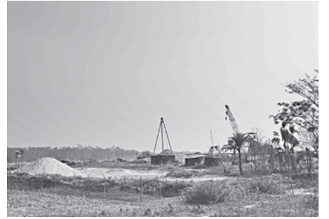
Except for a few equipment and some construction materials in Kalakhali village in Pirojpur Sadar upazila, on the bank of the Kaliganga river, no significant sign of development or activity was found as part of the ongoing work to build the bridge between Pirojpur Sadar and Nesarabad upazilas. The photo was taken in last week of December last year. PHOTO: STAR
